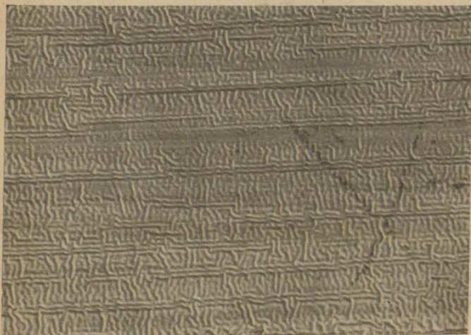
FIGURE 22.— Paint that has wrinkled soon after application.
